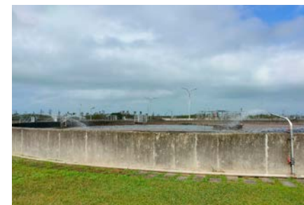
De-foaming Water from Secondary Clarifiers
