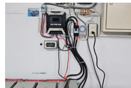
Components of Energy Storage Device
