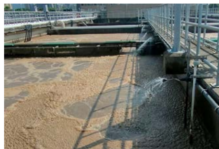
De-foaming Water from Aeration Tanks
